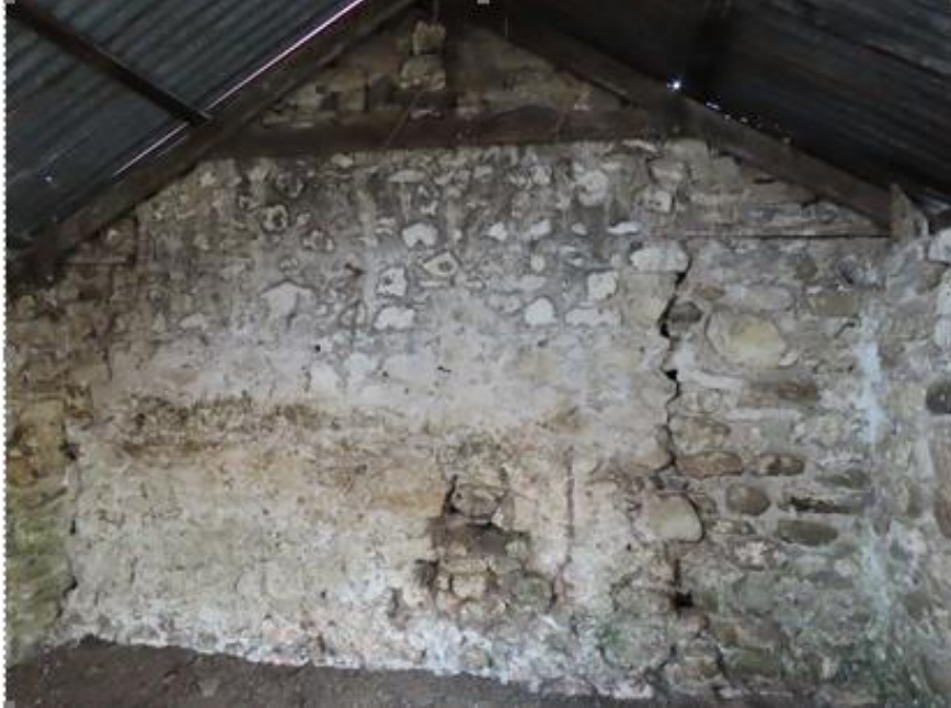
Photo 20 – crack in stonework of gable wall – ideal roosting site for bats
