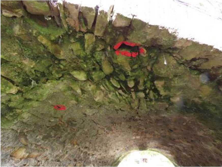
Photo 10 – two crevices marked for retention for bats close to downstream face of eastern arch
