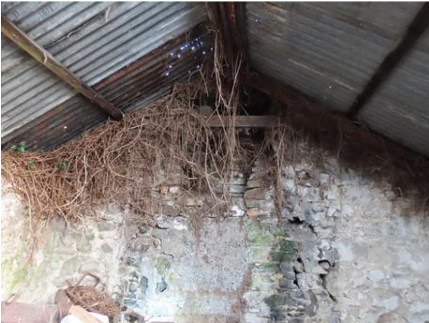
Photo 21 - crack in stonework of gable wall – ideal roosting site for bats
