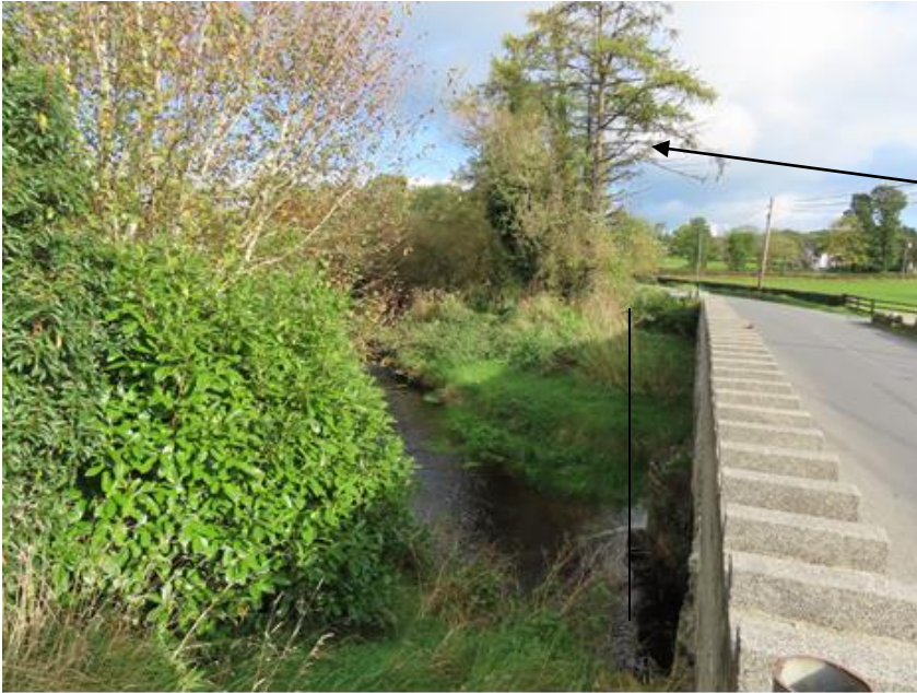
Photo 4 - position of proposed walkway to north of bridge structure (upstream). Several conifer (fir) trees to be felled on east side of bridge
