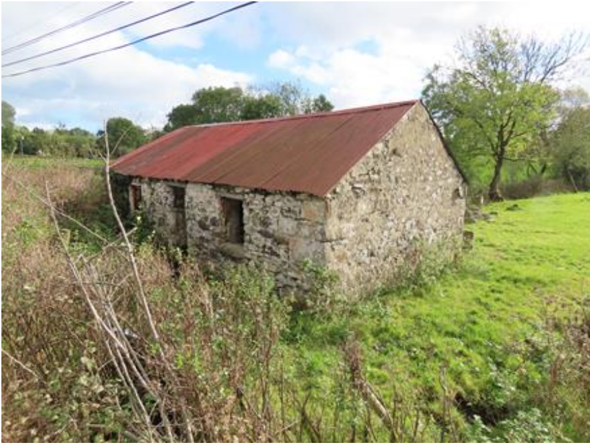
Photo 18 – farm shed on western side of river which will be demolished to accommodate road widening
