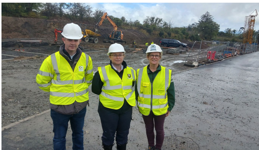
September 2025: On-site Building Control inspection, in conjunction with the National Building Control Office (NBCO)
