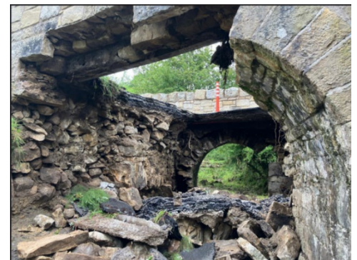
Above: After Flood Damage
