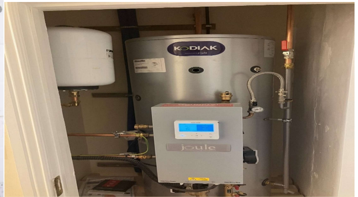
Example of Integrated HP Unit installed
