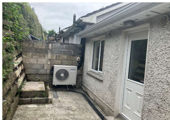
Heat Pump Unit fitted at OPD Dwelling
