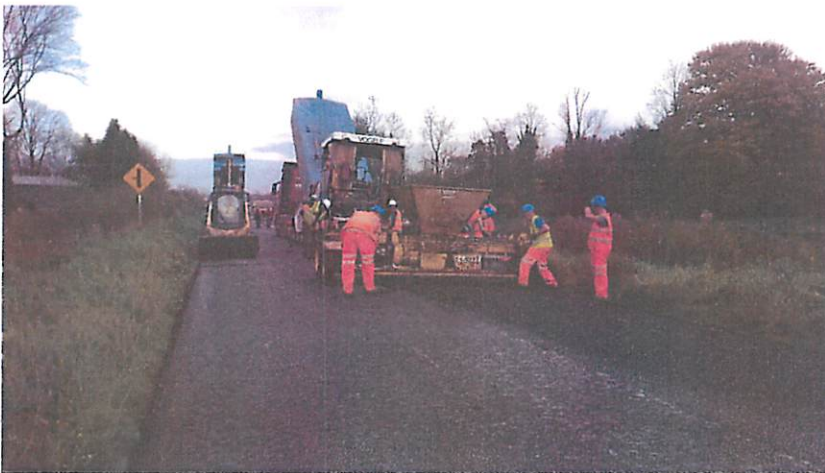
Photo showing Chip laying crew on the N87 Lisnamine to Rahaghan Pavement Overlay Scheme
